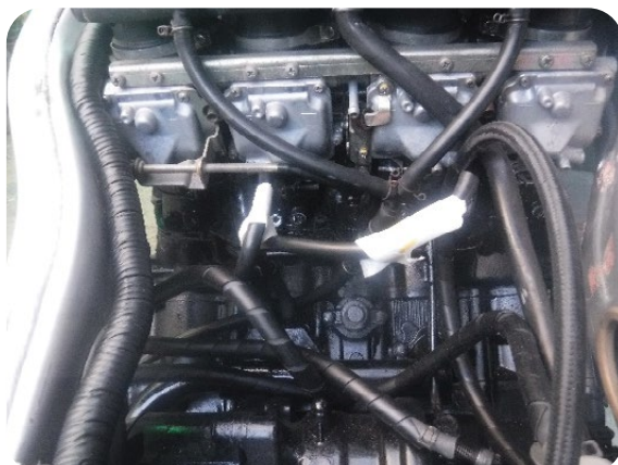
New piping and sparkplug leads
